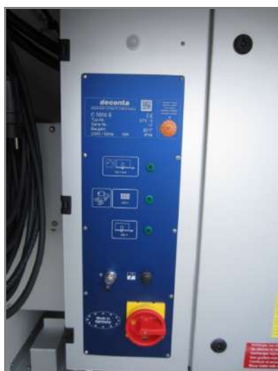
Fig. 1 16 Emergency shutdown switch
