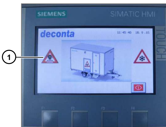
Fig. 1 67 Status of the alarm system
