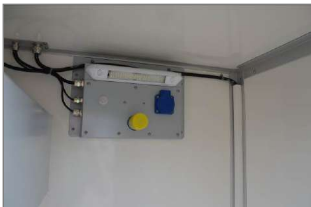
Fig. 1 126 Vacuum cleaner connection in additional chamber
