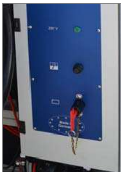
Fig. 1 17 Battery main switch
