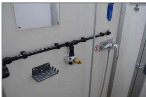
Fig. 1 125 Compressed air supply
